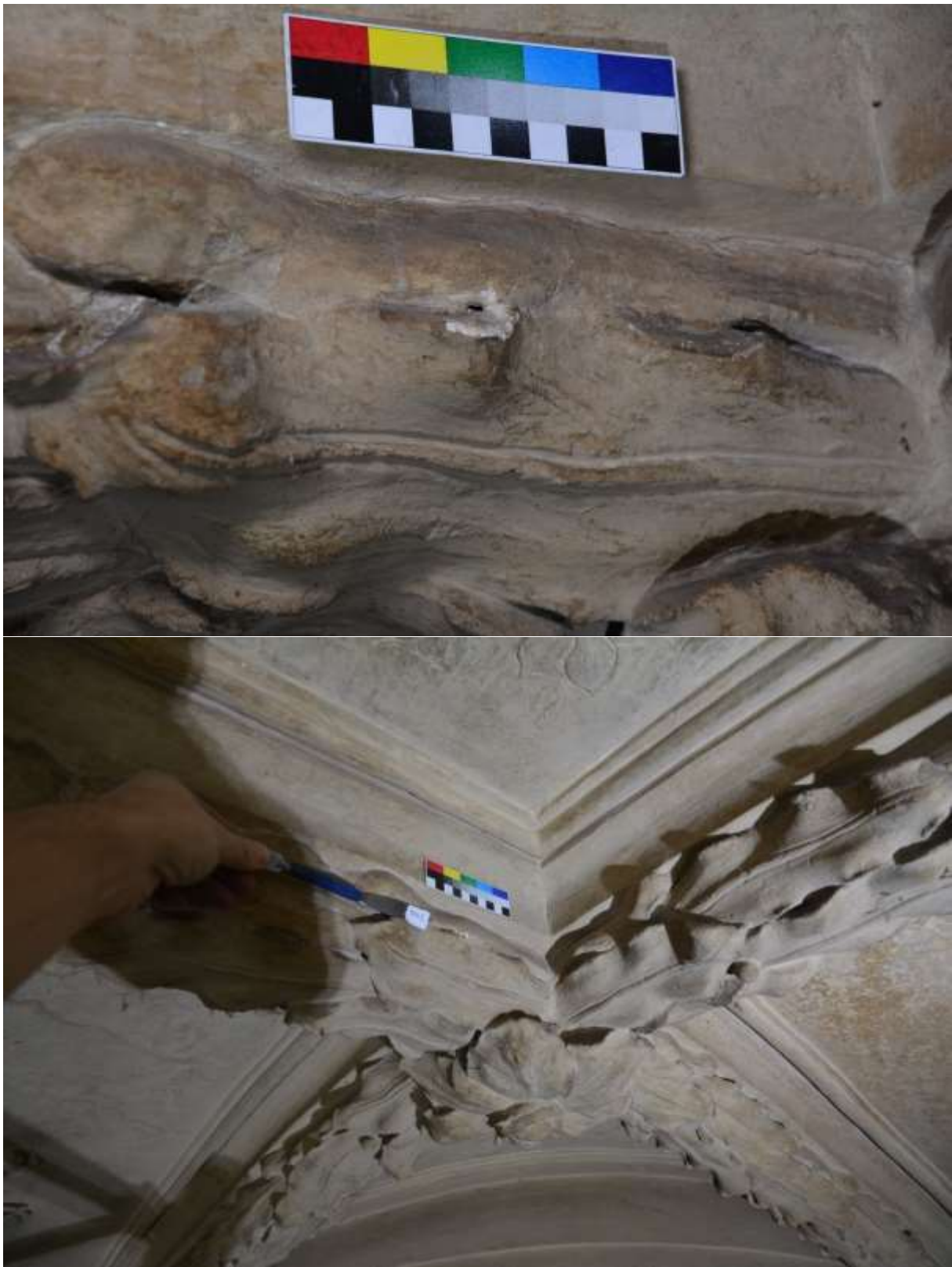
A fragment from a leaf covering the rib. Top section of the vault. The small fragments are detached from the main bulk of the rib.
