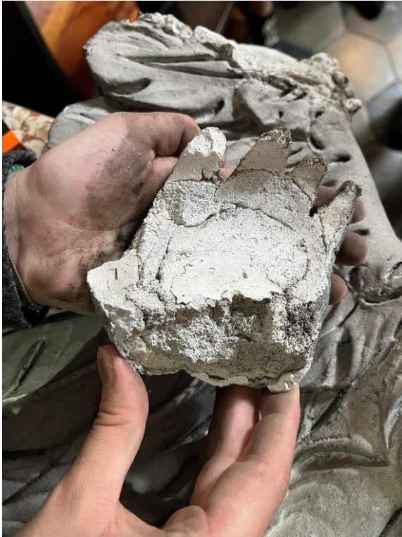
Fig. 13. Detached elements of stucco decoration make it possible to observe construction details such as the different layers of stucco mortar used for building up a hand.
